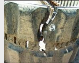
Steel cord breakage caused by de-tracking
