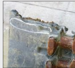
Steel cord breakage at end of overlap
