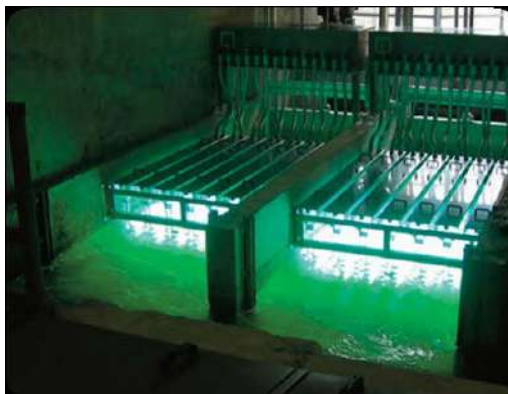
Savona wastewater treatment plant.
