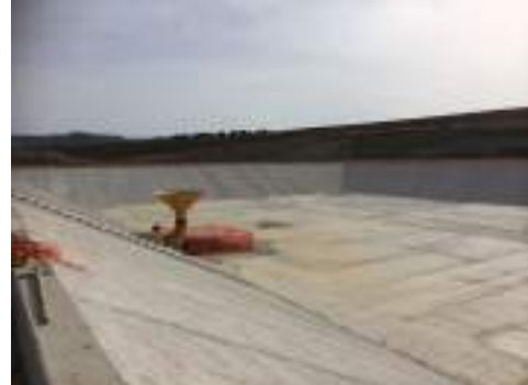
Detail of a basin
