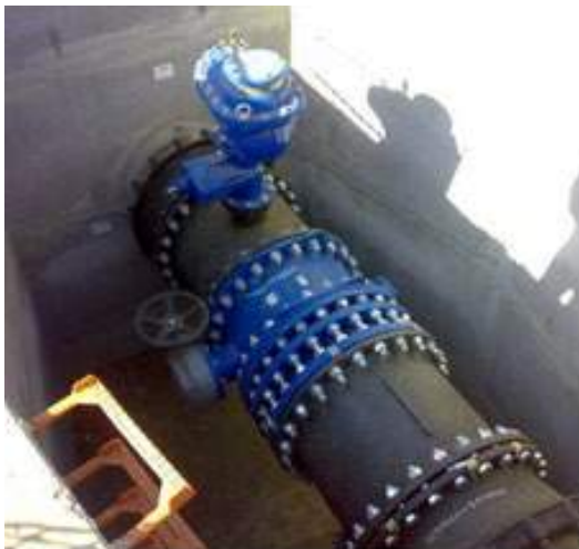
Detail of the main pipe
