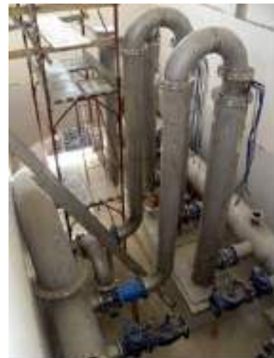
Detail of a pumping station
