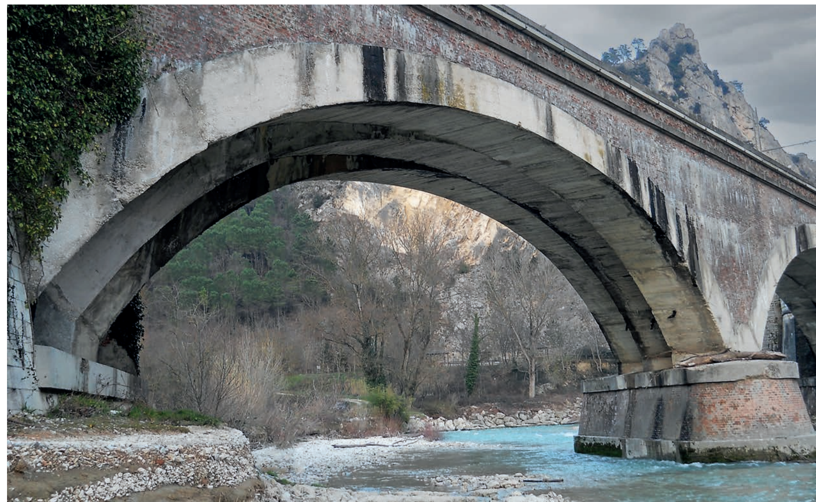
2. 3-blade masonry arch bridge with 2 spans. Above: structural reinforcements to ensure seismic suitability Below: state of affairs before construction
